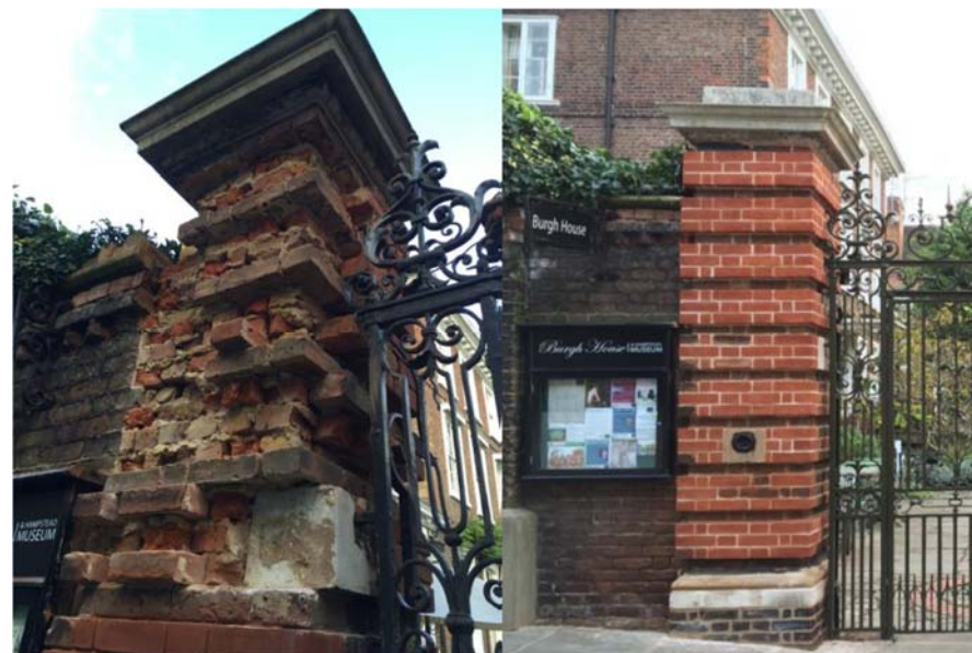
Above: Before and after - gate piers at Burgh House Below: refurbished staircase at Burgh House
